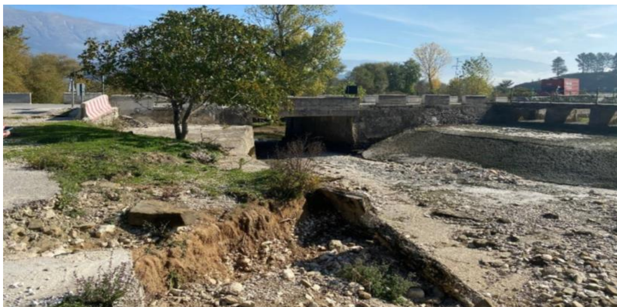
Figure 15: Damages to the structures and the lake bed after the high water levels.
